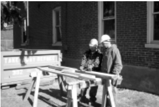
Foundation Board Member Johnny Figueroa (r) supervises a crew of five students at one of the sites on Freemont Street in Lancaster.
